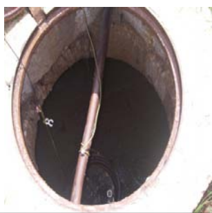
SS 1: at Equalization tank
